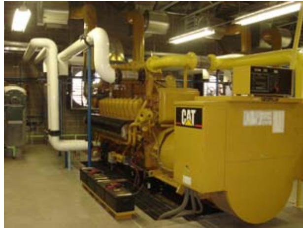
Figure 5: equipment for energy recovery from landfill gas.
